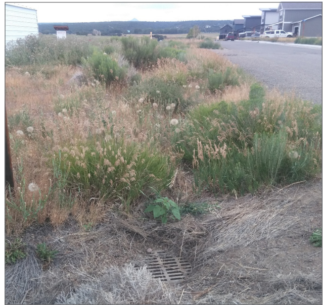
Figure 8-5: Clogged/Buried Inlets Along Pinion Street
