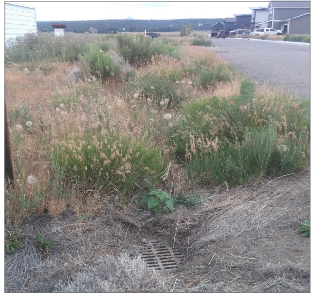
Figure 8-5: Clogged/Buried Inlets Along Pinion Street
