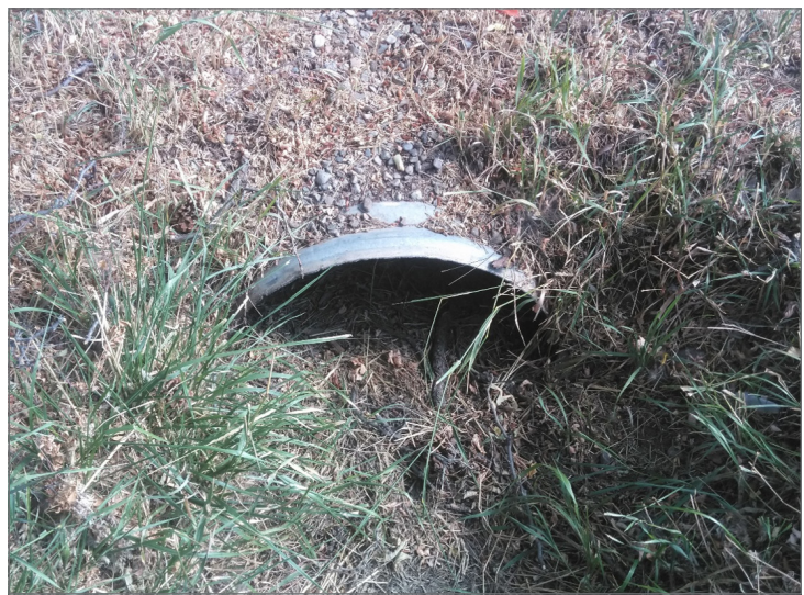
Figure 5-4: Culvert and Ditch with Debris and Sediment
