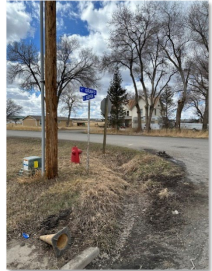
Aspen Street and CR Z42 / Grand Avenue intersection is a drainage problem area in the Town of Norwood.
